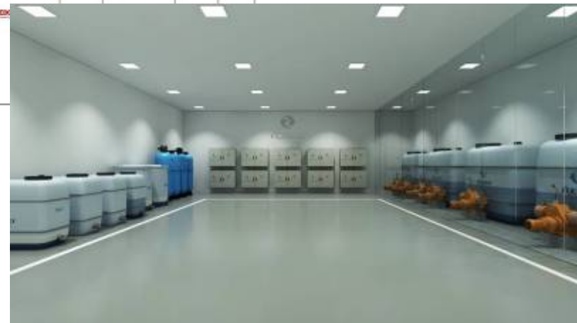
The Zagazig Water Treatment Station, Egypt. Contractor: Al-Eman Engineering Co. – Disinfection REDO - 17.000 m 3 /d
